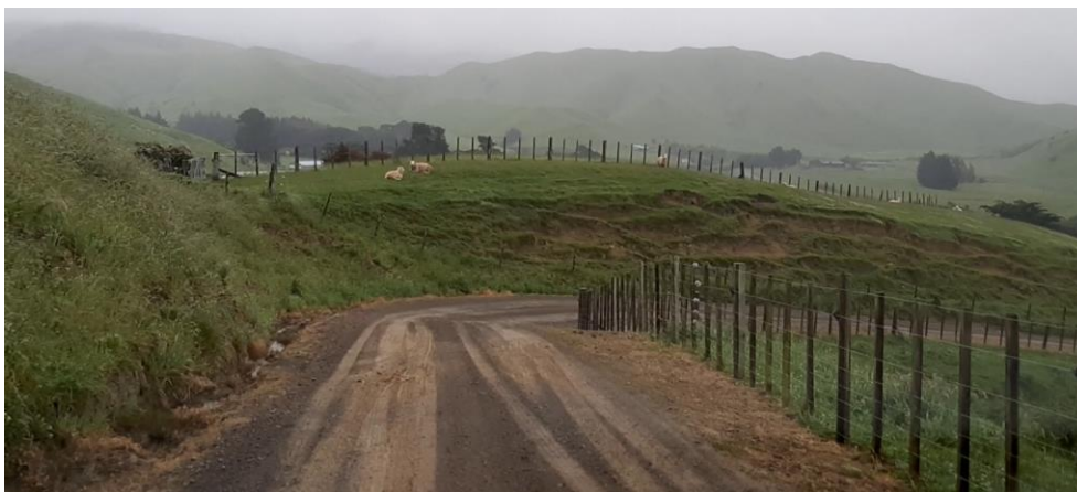
Figure 2.14: Example of poor grading on Coach Road South
